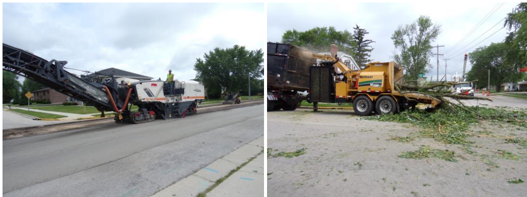
Pictured: Milling of asphalt and removal of street trees in phase I of Main St Project
